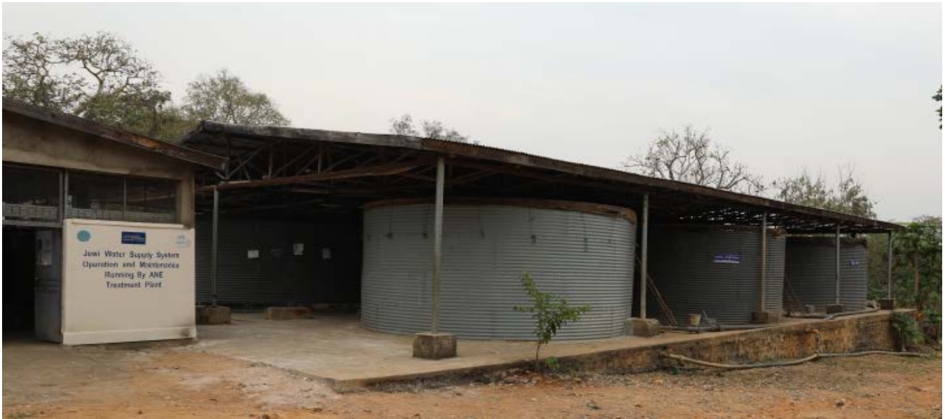
Jewi water supply system
